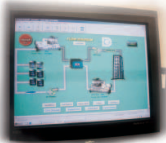
Chiller plant and ice storage operation are managed by Tracer Summit system.
